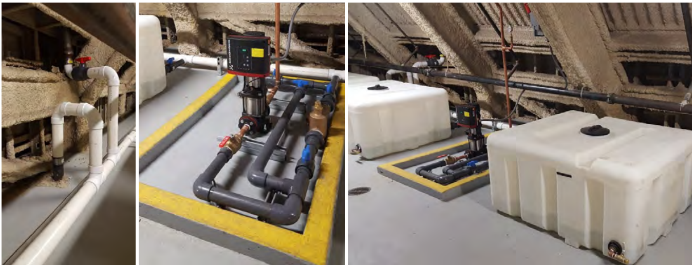
Pictured: Wright Runstad & Company's rainwater capture and reuse system at their 1201 3rd location in downtown Seattle. The engineering team at the site creatively solved their water challenges by piloting both groundwater and roofwater capture and reuse to offset the building's irrigation and cooling tower needs, collectively saving on average 864,000 gallons of water per year. The project was awarded the 2018 Vision Awards Water; more info can be found here .
